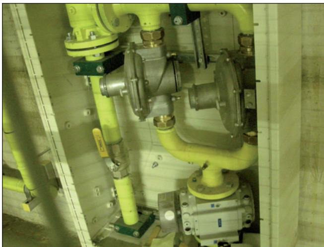
Natural Gas Meter supplying central plant. Bord Gáis Networks G65 meter supplying up to 1035 kW.
